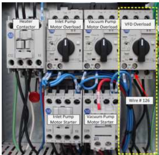
Outlet Pump Motor Drive Overload
